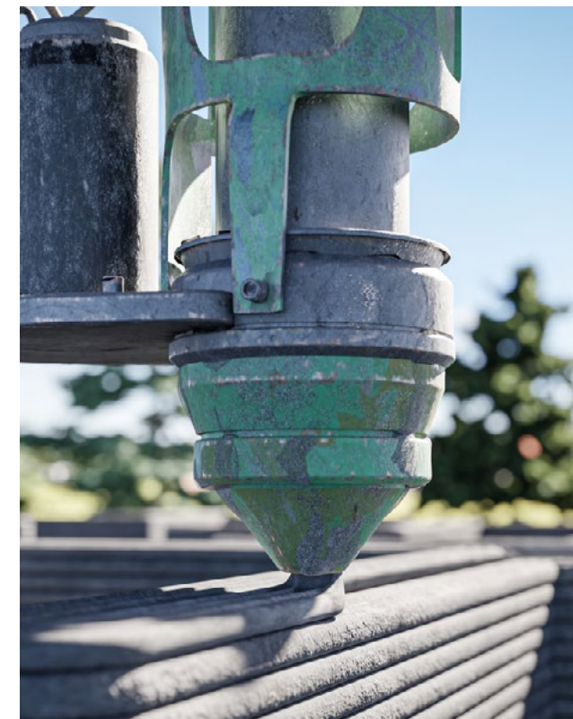
Companies are increasingly using materials such as clay and sawdust for the 3D printing of houses.
